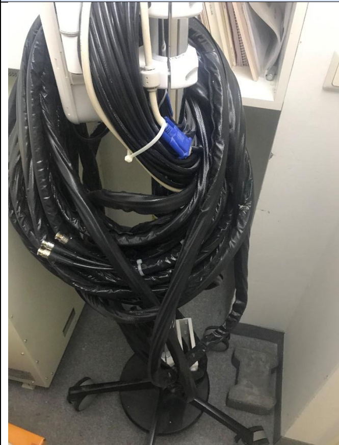
Spare In room Monitor Pedestal
